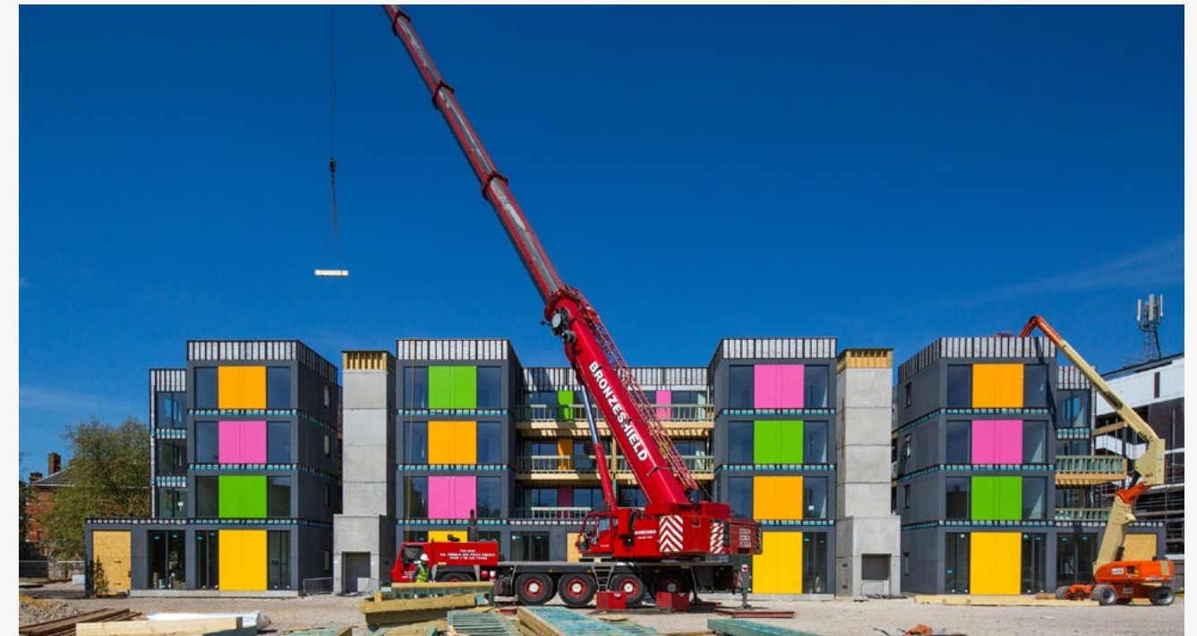
A modular future? — PLACE / Ladywell in Lewisham by Rogers Stirk Harbour + Partners, AECOM and SIG
